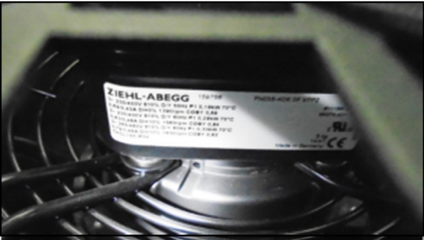
Photo #7 Test unit condenser fan
