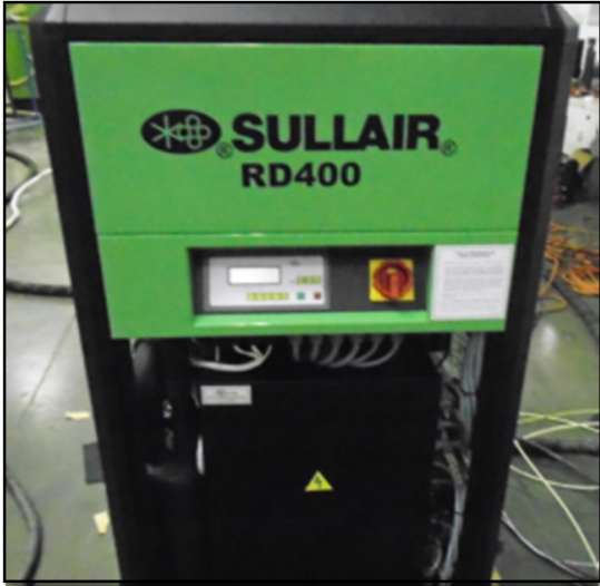
Photo #6 Test unit set-up
