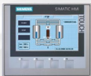
Touch Screen PLC - Pic. 2
