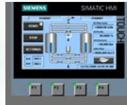
Touch Screen PLC
