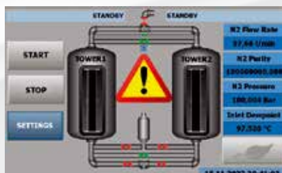
Touch Screen PLC - Pic. 2
