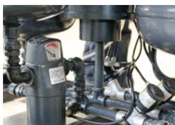
Air Filter - Pic. 5
