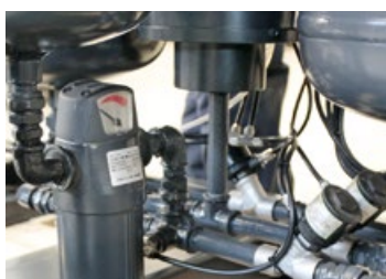
Air Filter - Pic. 5
