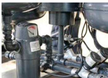
Air Filter - Pic. 5
